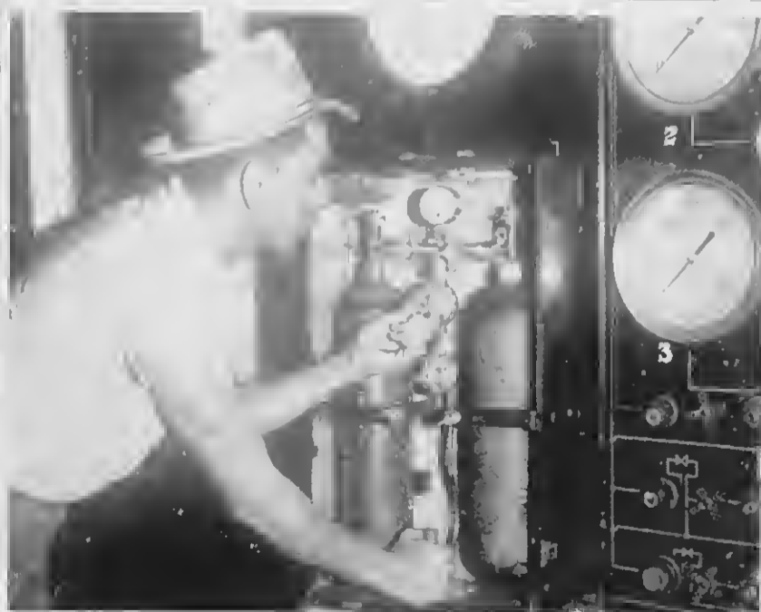
WHILE THOUSANDS of men busied themselves with the processing of oil Dec. 31, Instrumentman Antero Dykhoff quietly concentrated on a humanitarian deed. His was the project of repairing a valve on oxygen bottles used for the San Pedro Hospital incubators. The valve was repaired and returned to the hospital — a small deed quietly done in the heart of the world's largest refinery as an aid to the community in which it operates.
